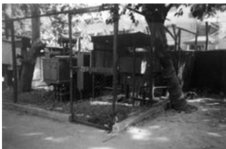
Fig. B39 : Outdoor substations without enclosures
