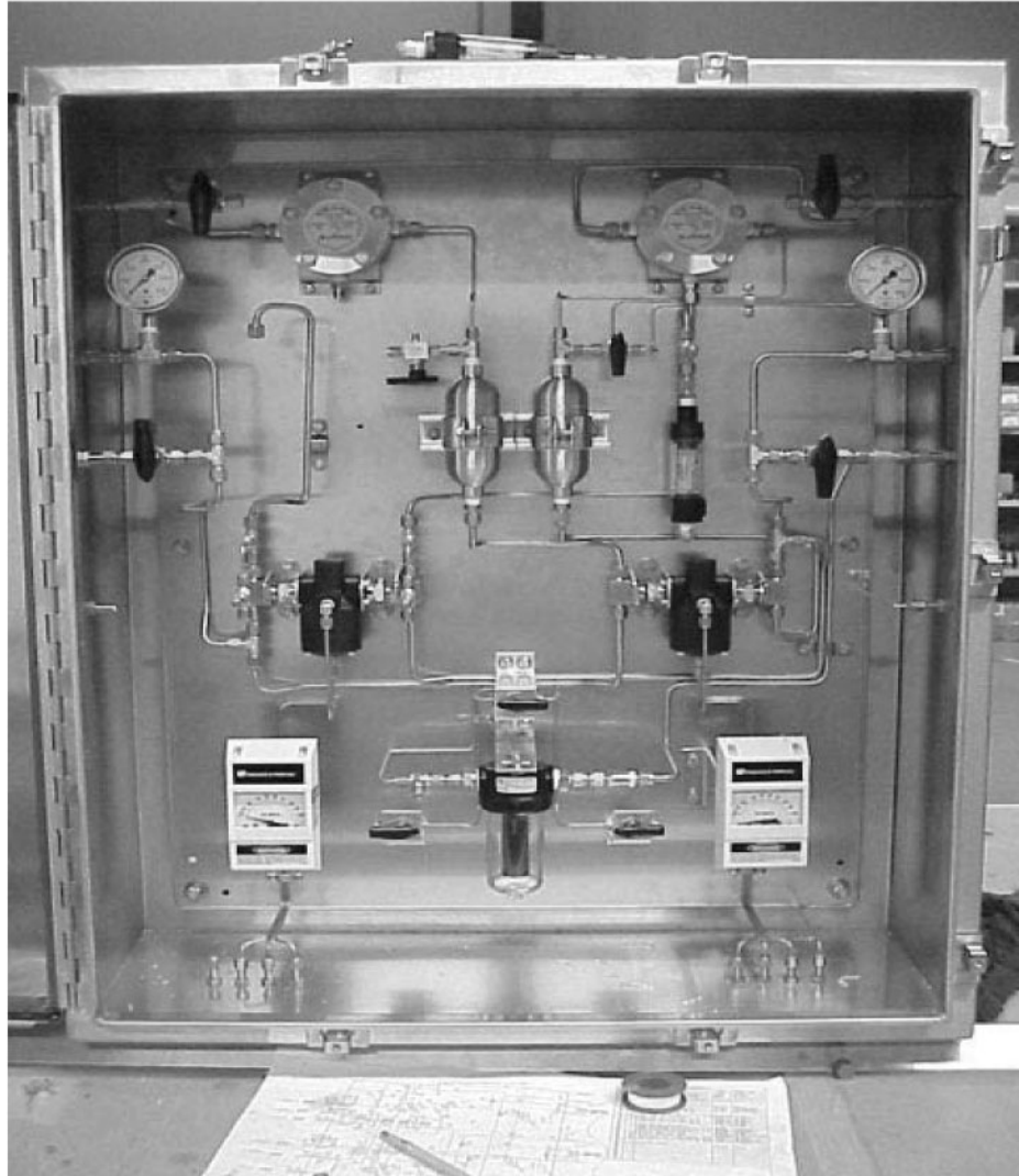
Figure 2-1: Example of a Boxed Sampling System (Courtesy of Technical Automation Service Corp. [TASC])
