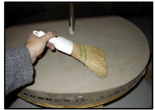
Flywheel is poured in form made by tacking tar paper to plywood disk. Partly set concrete is "broom-finished."
