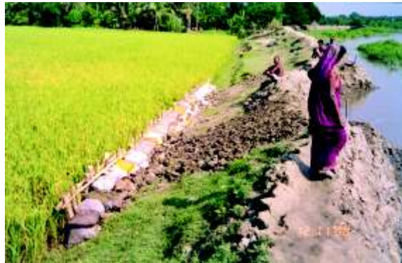
Photo 4.2: Embankment on the verge of collapse
